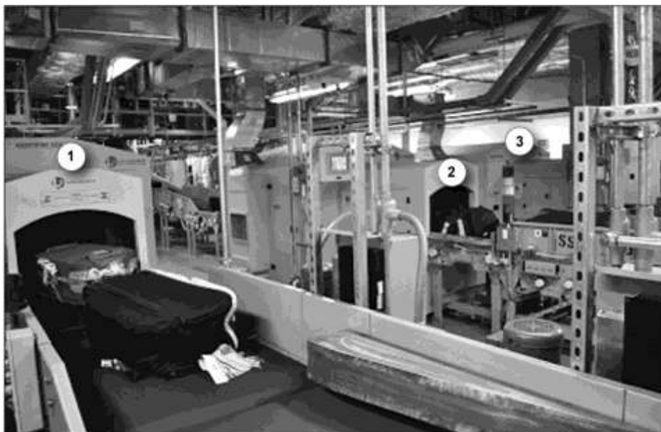
Figure 1 - A Checked Baggage Inspection System that Includes a Baggage handling System (BHS) with three in-line EDS Machines
